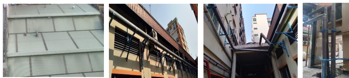
Pic4: Pipe networking and Storage
